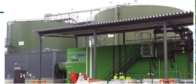
FPBO storage at Empyro (250 m 3 )
