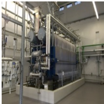
Production of hydrogen in 6 MW electrolysis
